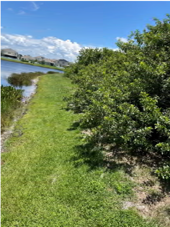
Location 20: Invasive vegetation growing onto pond berm. Remove approximately 5'x250' of vegetation to prevent turf deterioration/erosion.
