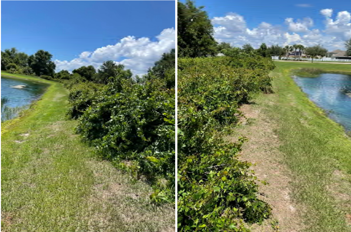
Location 19: Invasive vegetation growing onto pond berm. Remove approximately 5'x250' of vegetation to prevent turf deterioration/erosion.
